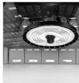
Indoor Low/High-bay Application
